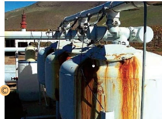
Filters are not functioning appropriately
